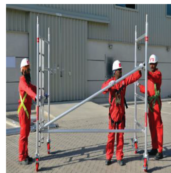
3 Fix the diagonal braces from the bottom of the first frame to the third rung and repeat the same for all frames.
