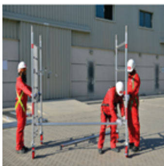
2 Fix the horizontal braces on the end of both frames to get stability and repeat the same for all frames.
