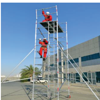
10 Fix the horizontal braces on guardrail similar to ones shown before and fix the toe board.
